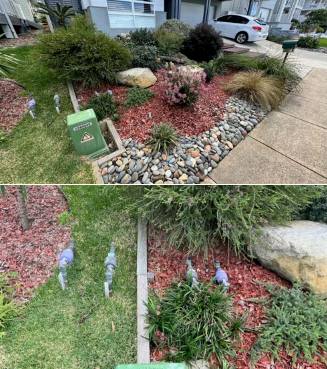
Figure 6. Established (Stage 1) property meters (9 Anouska Street) showing intact water and lilac-coloured recycled water connections.
