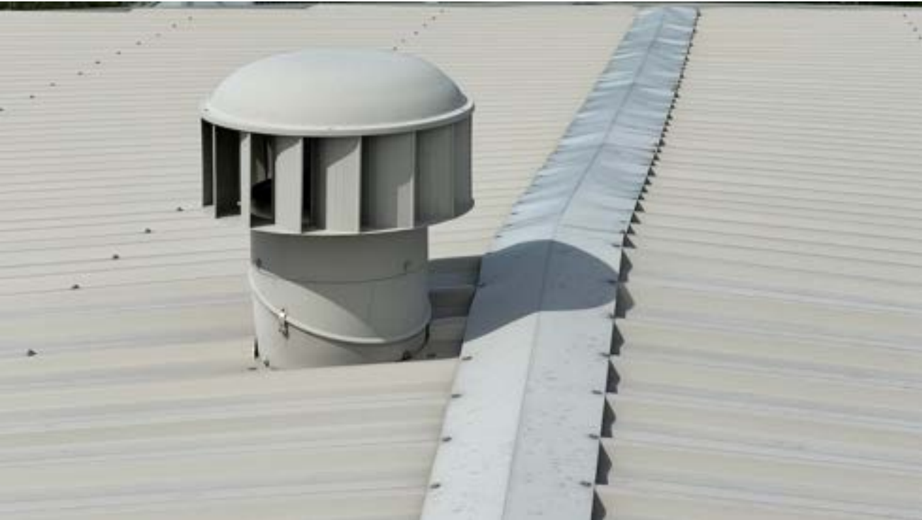
Figure 3. Intact and functional vent on treated drinking water storage tank, in good condition.
