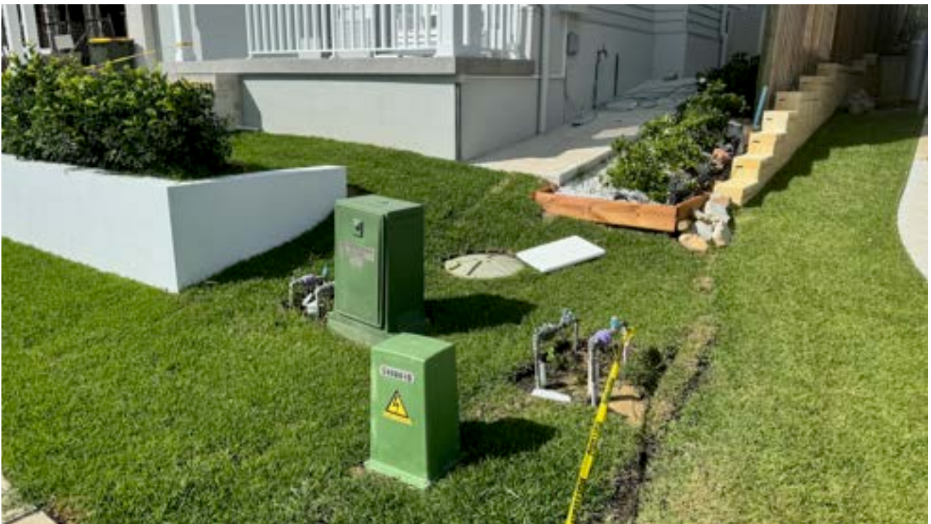
Figure 8. Established Stage 6 (2021) connection (13-15 Hopwood Close) showing intact and accessible structures and lilac-coloured recycled water.
