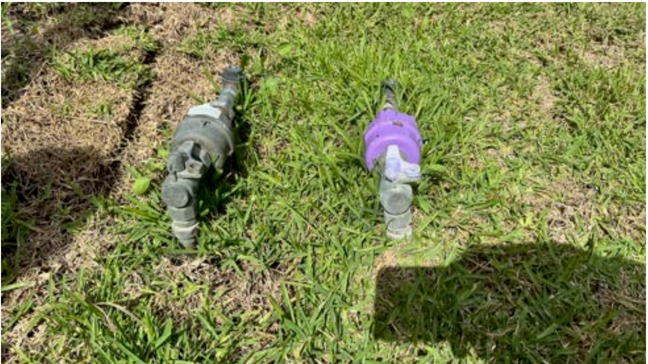
Figure 5. Established Stage 7 property meters (30 Raywood Circuit) showing intact water and lilac-coloured recycled water connections.
