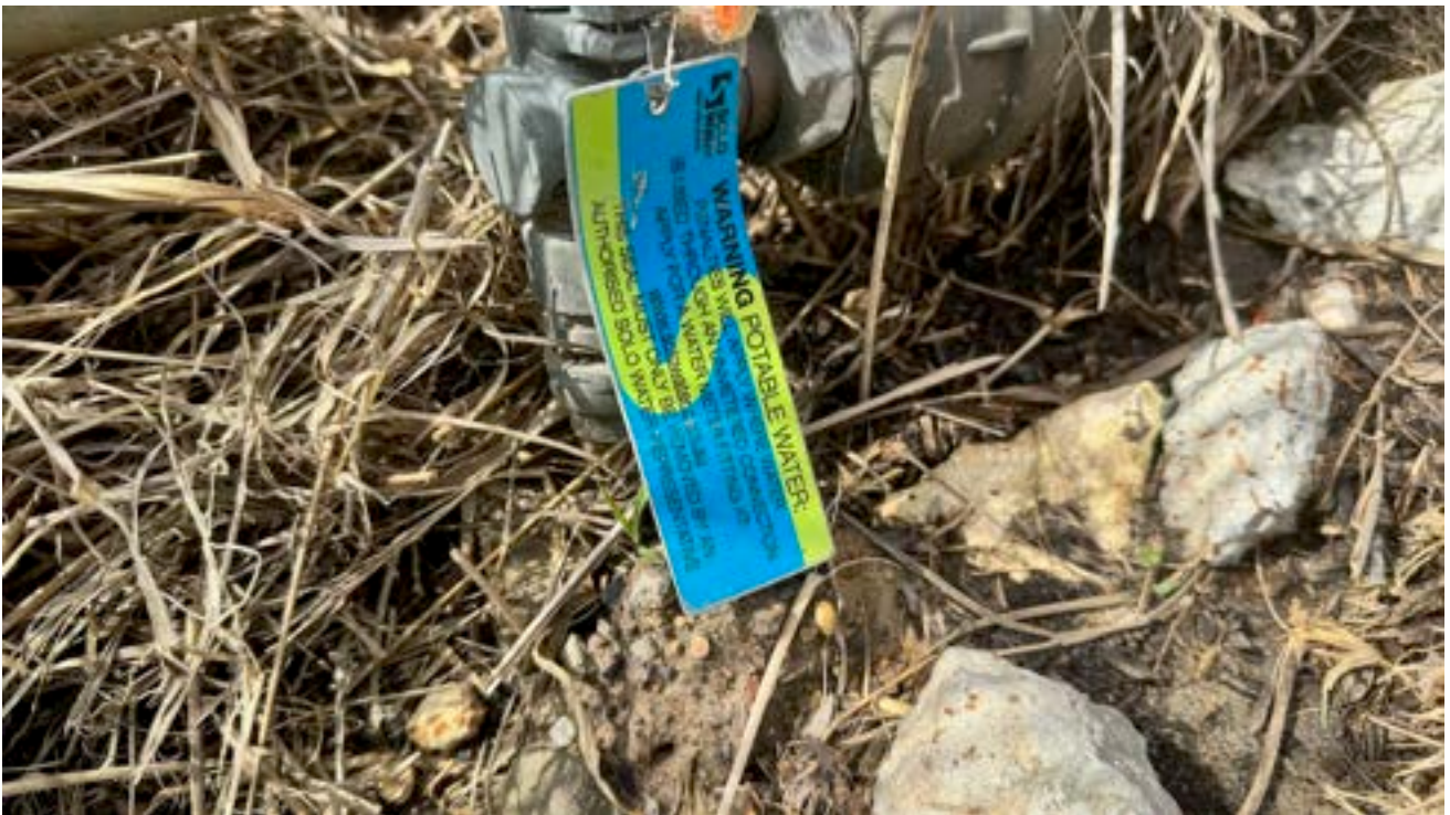
Figure 9. New connection (32 Raywood Circuit) showing locking pin on recycled water and feed from potable system.
