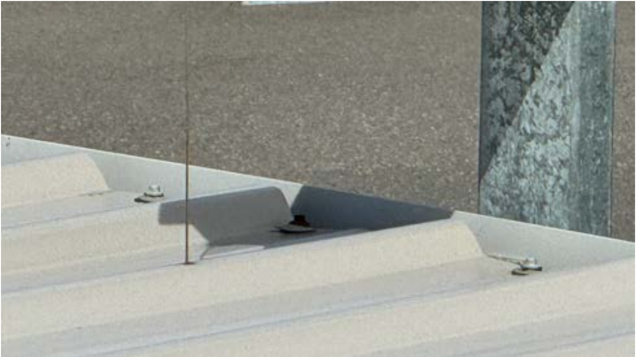
Figure 4. Level sensor entry point on treated drinking water storage tank – this was the only visible entry point.
